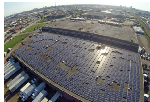
600 kW DC FIT 2 Project located in Brampton, Ontario, completed in July 2015.
