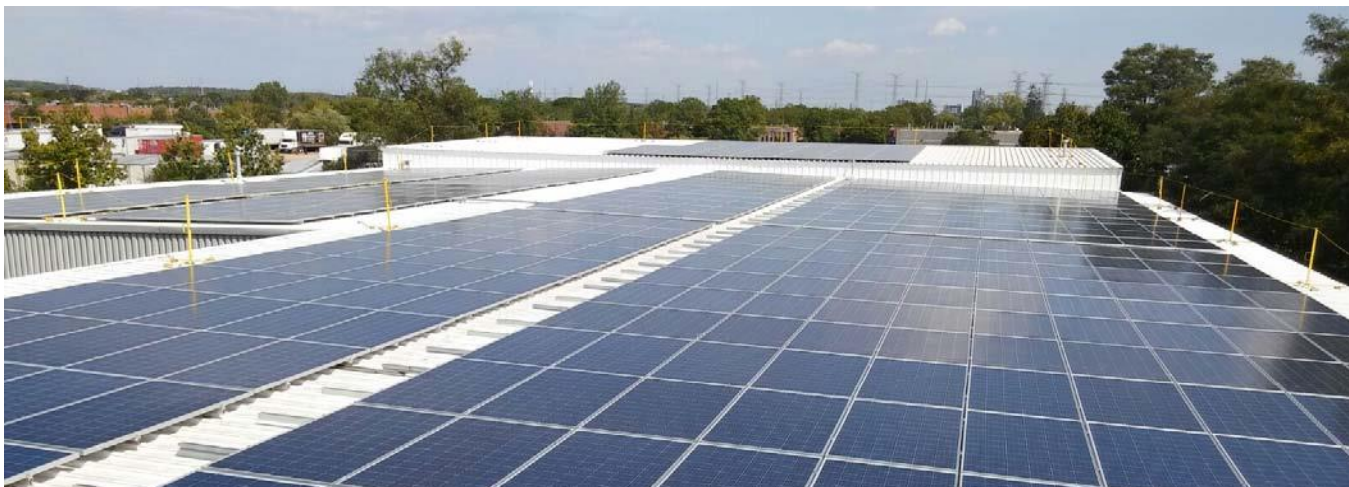
180 Kw FIT 3.1 Rooftop Project located in Vaughan Ontario.
