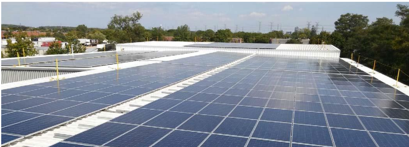
180 Kw DC FIT 3.1 rooftop project located in Vaughan Ontario.
