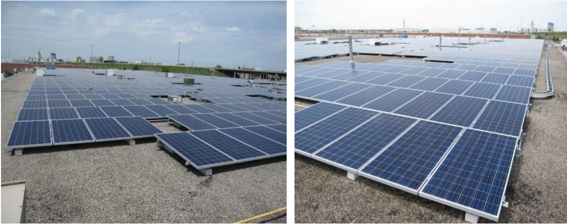
A 600 kW DC commercial rooftop project brought online last quarter.
