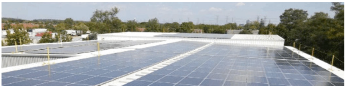
180 Kw FIT 3.1 Rooftop Project located in Vaughan Ontario Canada.
