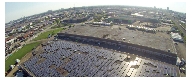
600 kW DC FIT 2 Project located in Brampton, Ontario, completed in July 2015.
