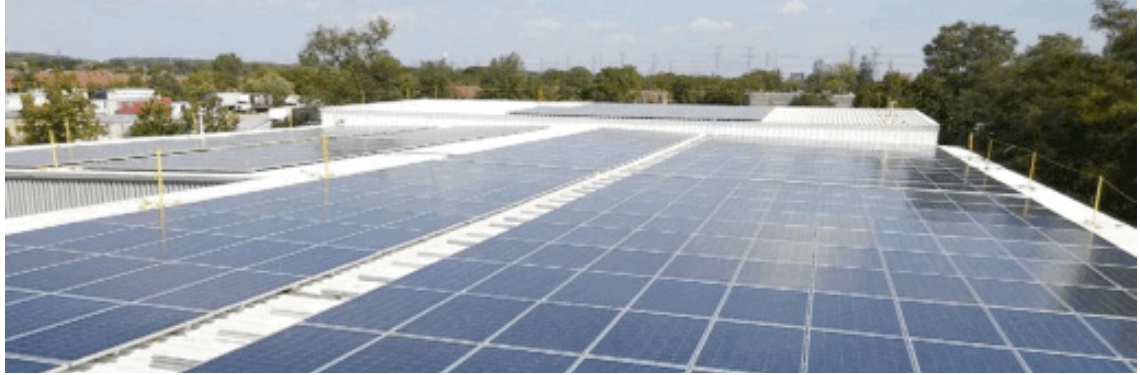
180 Kw DC FIT 3.1 Rooftop Project located in Vaughan Ontario Canada.
