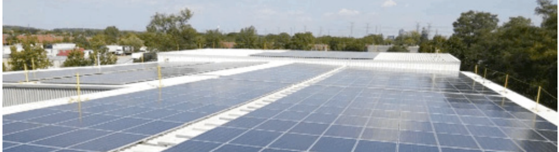
180 Kw DC FIT 3.1 Rooftop Project located in Vaughan Ontario Canada.
