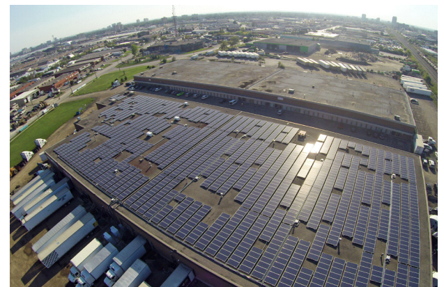
600 kW DC FIT 2 Project located in Brampton, Ontario, completed in July 2015.
