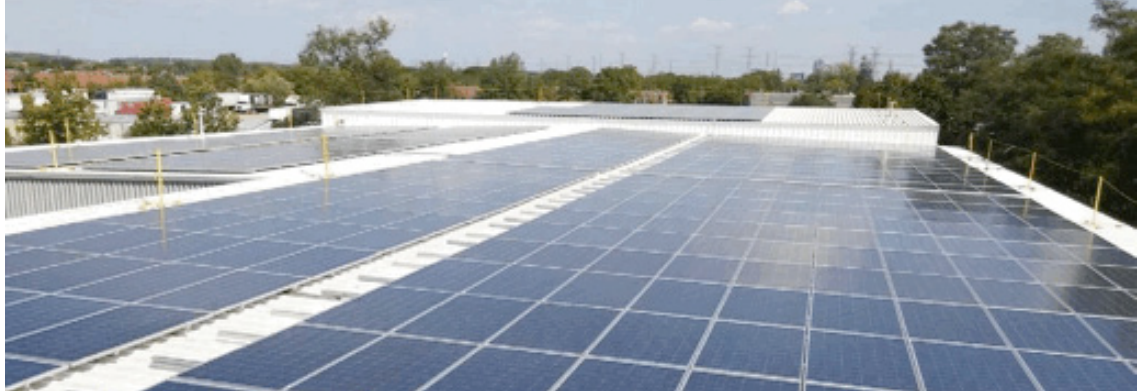
180 Kw DC FIT 3.1 Rooftop Project located in Vaughan Ontario Canada.
