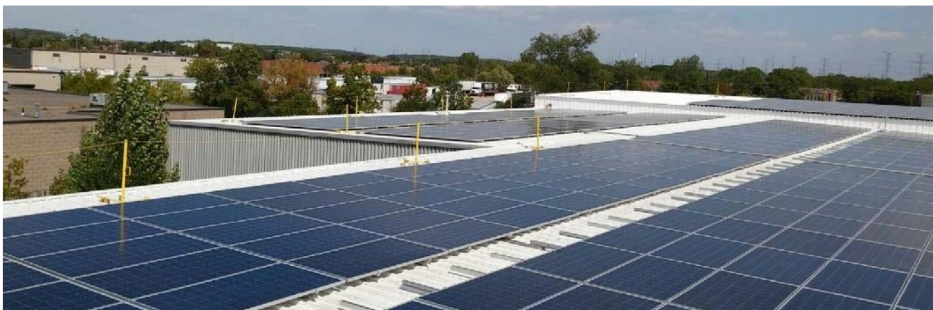
180 Kw FIT 3.1 Rooftop Project located in Vaughan Ontario.
