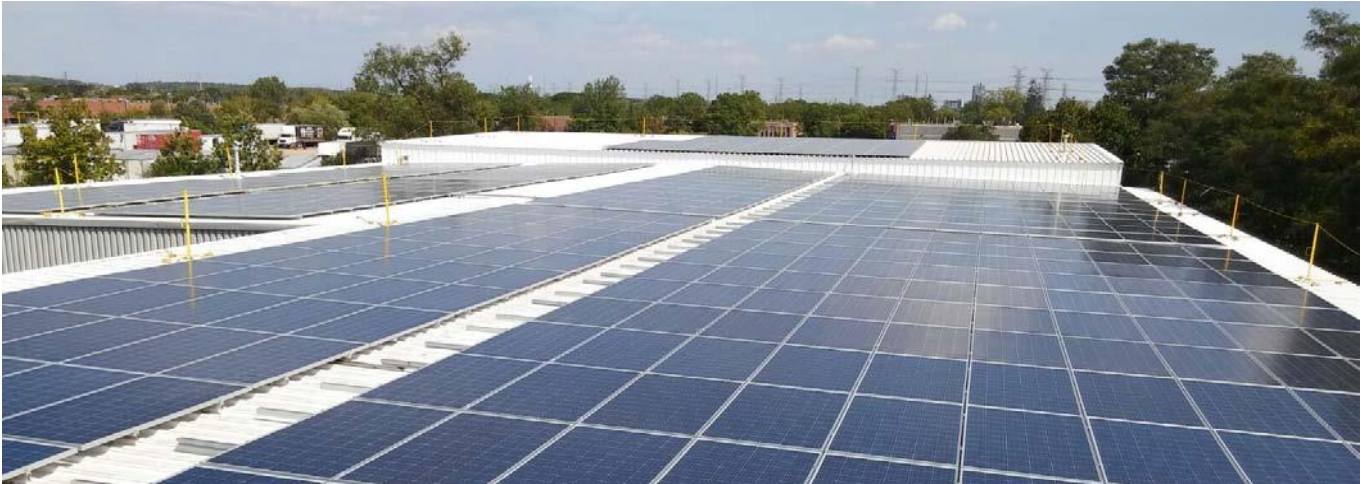
180 Kw FIT 3.1 Rooftop Project located in Vaughan Ontario.
