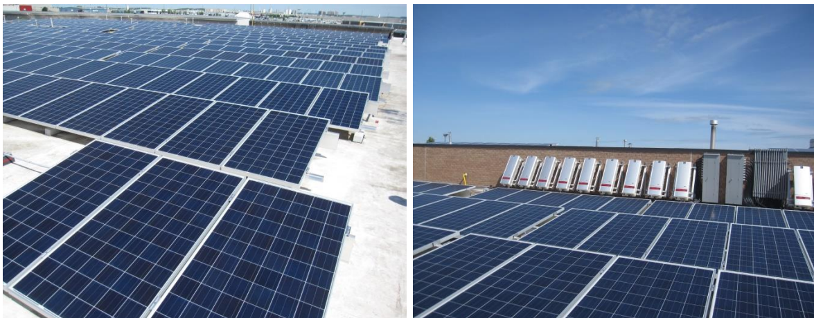
Shots of one of the 2012 LP's 235 kW DC commercial rooftop projects brought online in early June.
