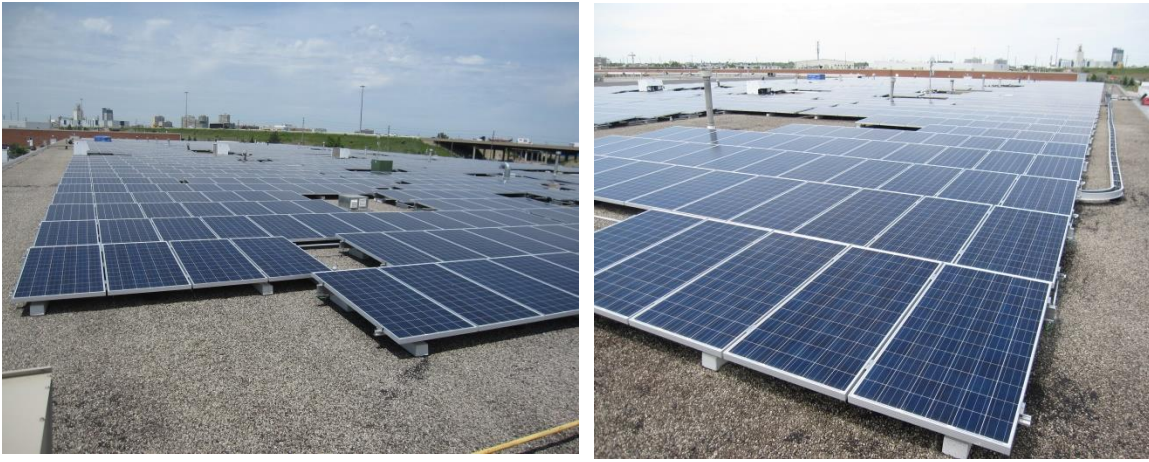
Shots of one of the 2012 LP's 600 kW DC commercial rooftop projects brought online in early June.
