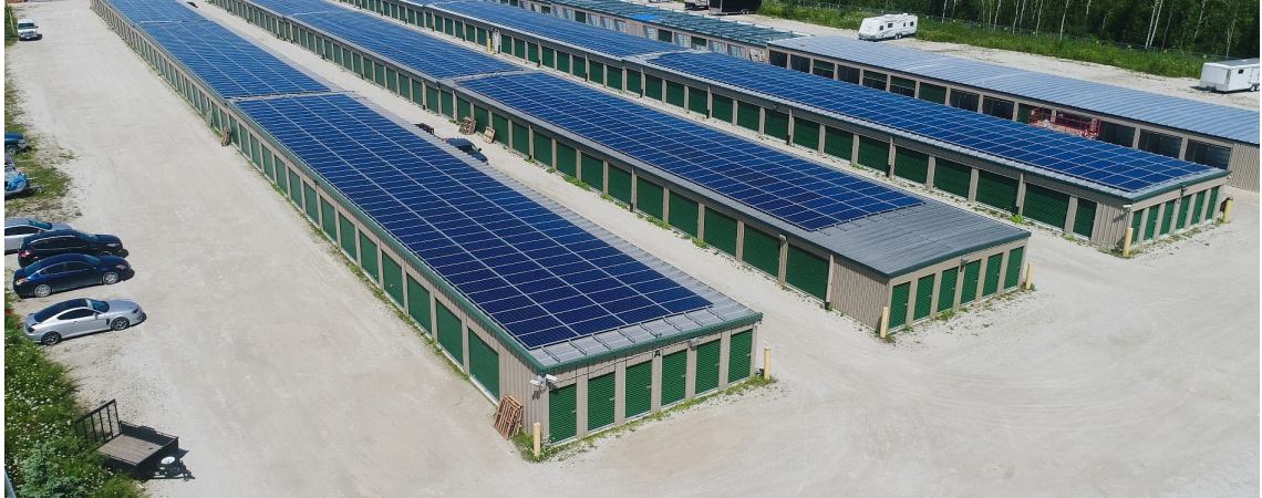
400 kW DC FIT 3.1 Rooftop Project located in Wasaga Beach, Ontario.
