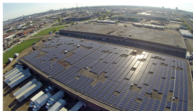
600 kW DC FIT 2 Project located in Brampton, Ontario, completed in July 2015.
