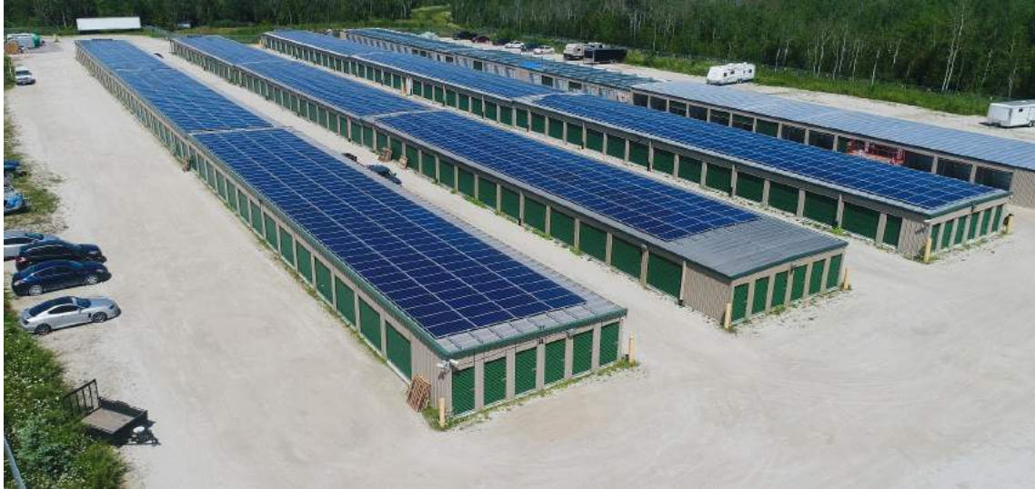
400 kW DC FIT 3.1 Rooftop Project located in Wasaga Beach, Ontario.
