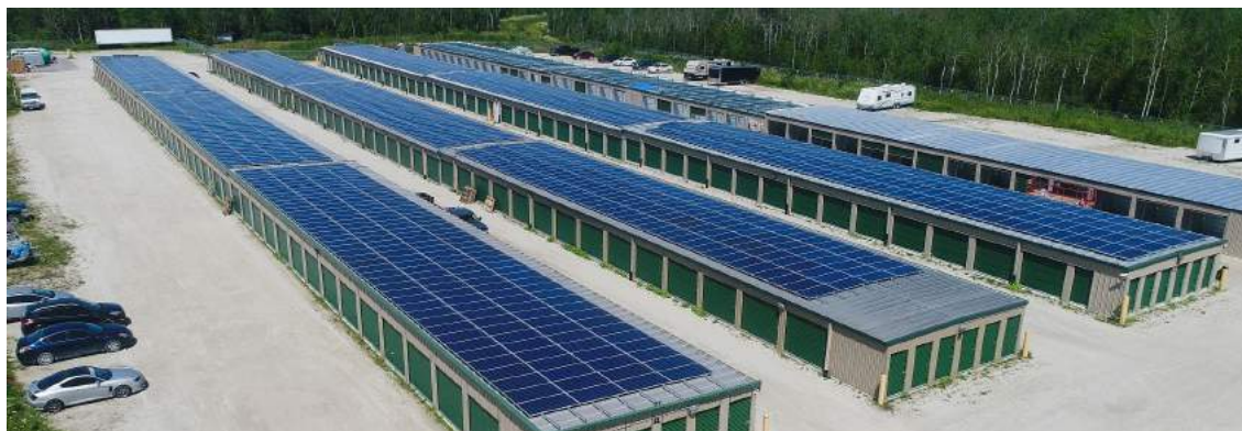
400 kW DC FIT 3.1 Rooftop Project located in Wasaga Beach, Ontario.
