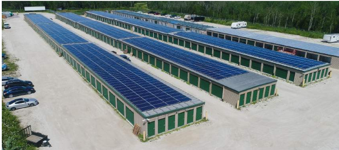
400 kW DC FIT 3.1 Rooftop Project located in Wasaga Beach, Ontario.
