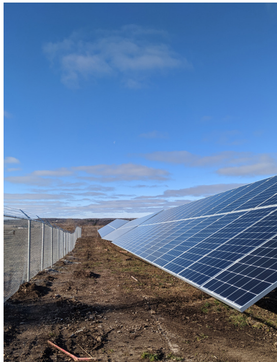
Project MS O5, a 600kW AC project completed in November 2020.
