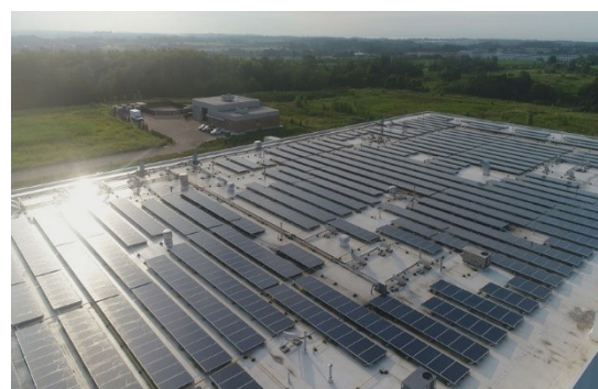
600 kW DC FIT 2 Project located in Ajax, Ontario, completed in July 2015.
