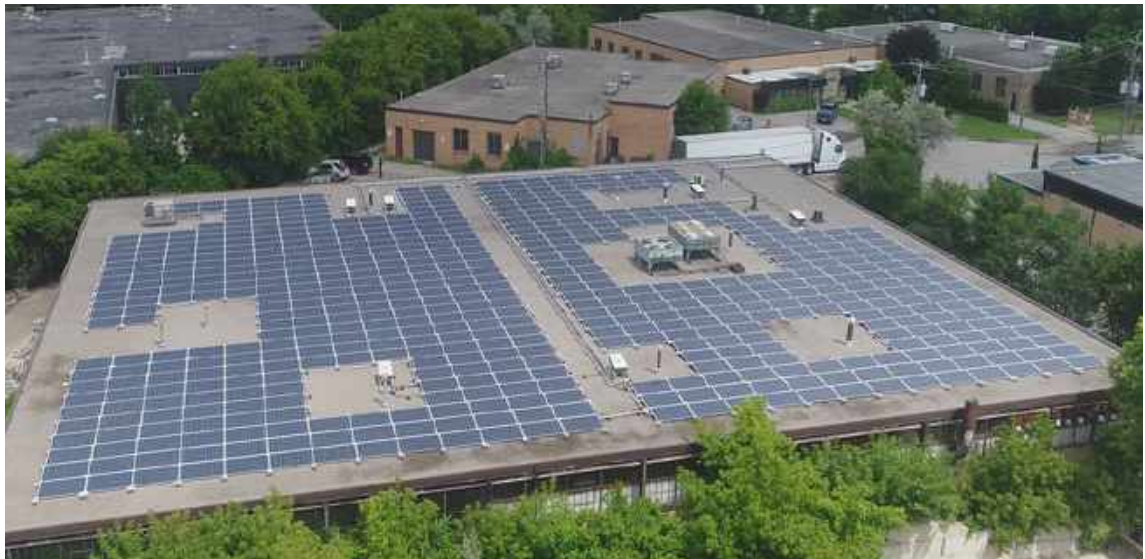
180 kW DC FIT 2 Rooftop project located in Toronto, Ontario.
