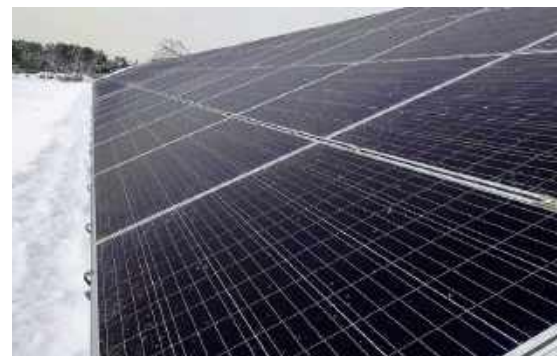
600 kW DC FIT 3.1 Ground Mount Project located near Newburgh, Ontario.
